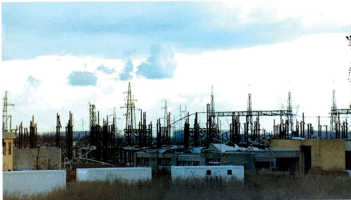
▽ Razorena transformatorska stanica Ernestinovo
