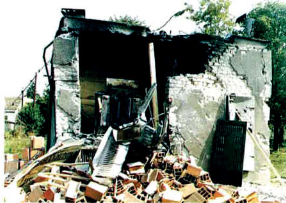
▼ Slavonski Brod - razorena transformatorska stanica Masarikova
