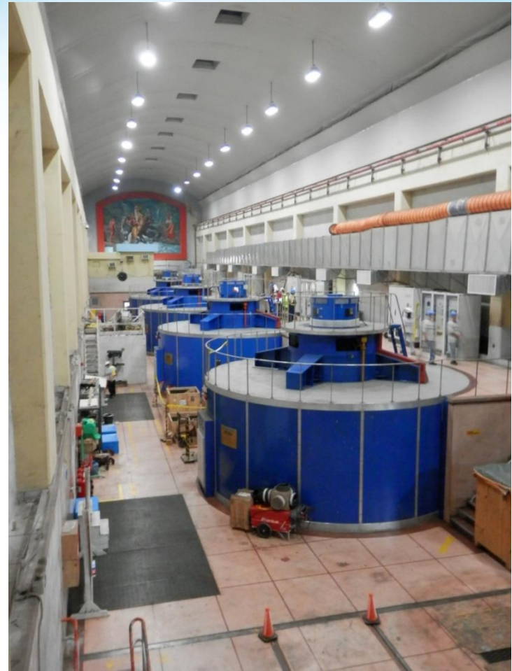
Generator za HE Binga
