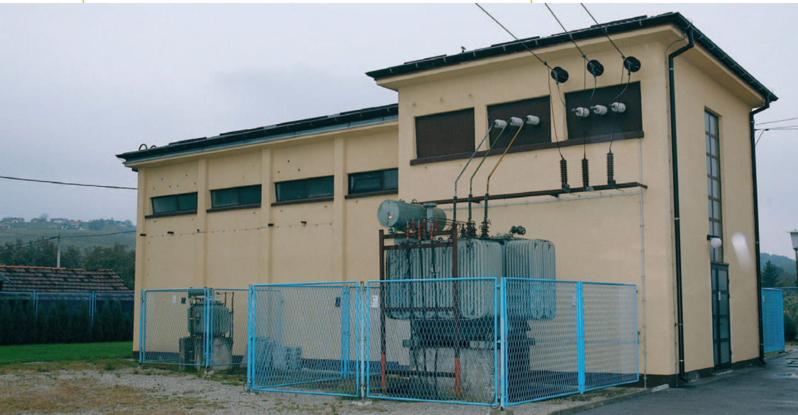
Transformatorska stanica 35/10 kV Vinica
