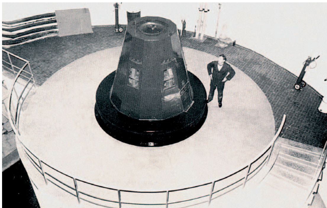
Generator HE Sklope
