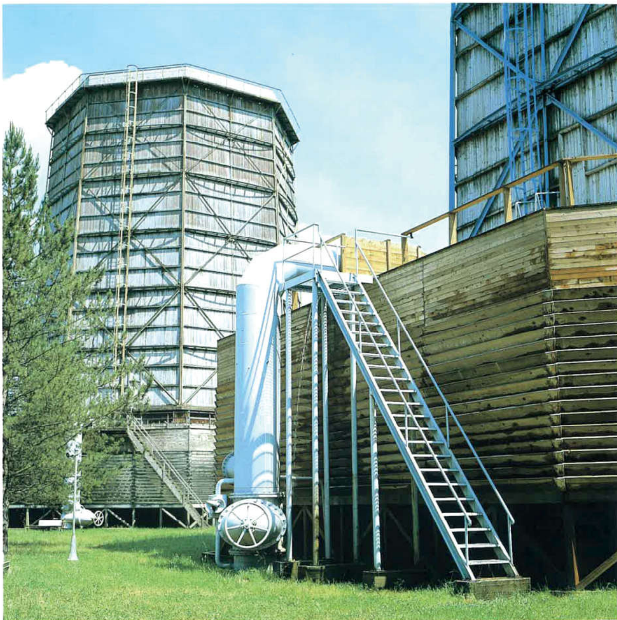
△ Cooling towers, the Jertovec thermal power plant
