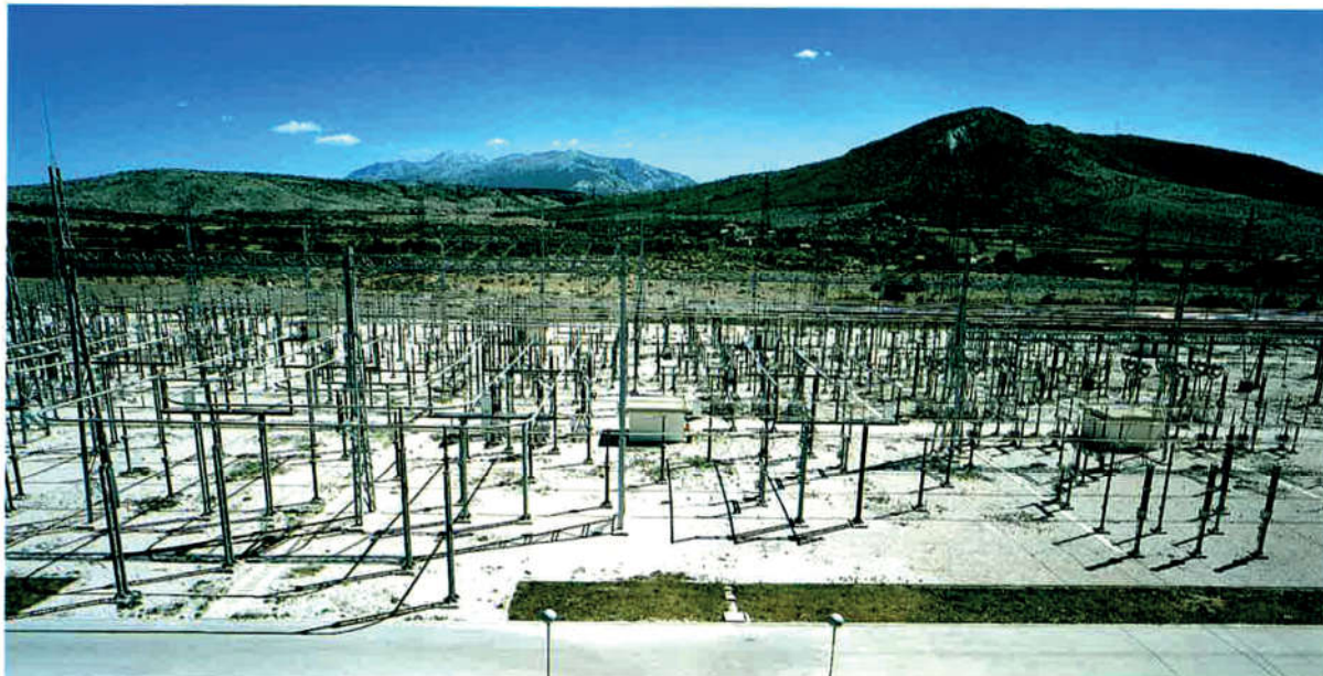
▽ The 400/220/110 kV Konjsko substation, near Split
