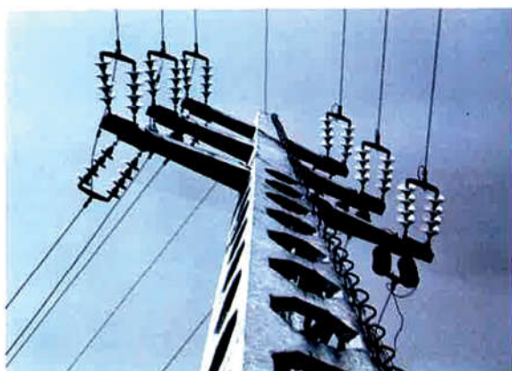
△ A concrete pole carrying the 30 kV double-circuit line Zagreb - Karlovac
