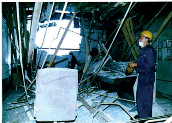
▽ Damage to the Osijek combined heat and power plant
