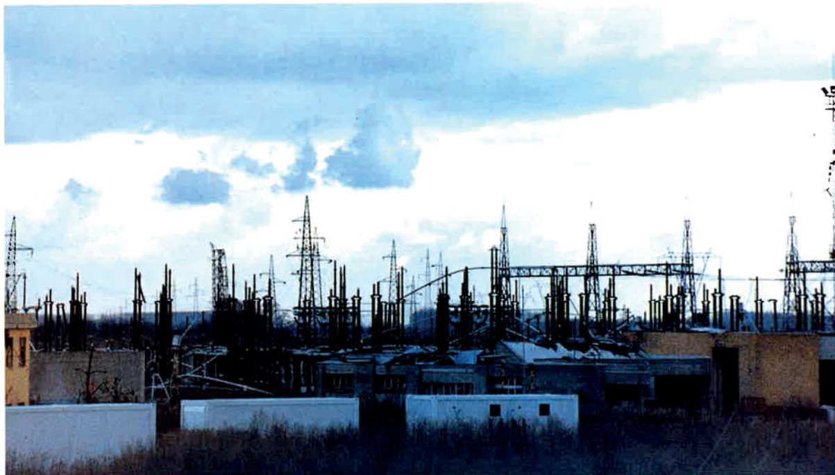
▼ Damaged and destroyed Ernestinovo substation
