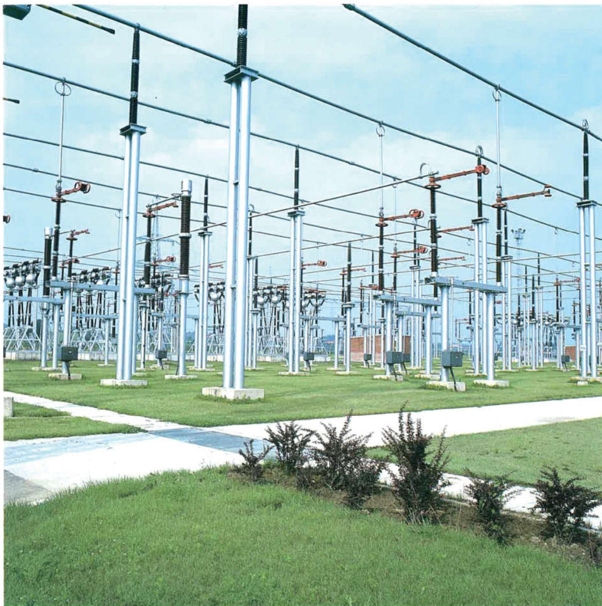
△ The 400/110 kV Tumbri substation
