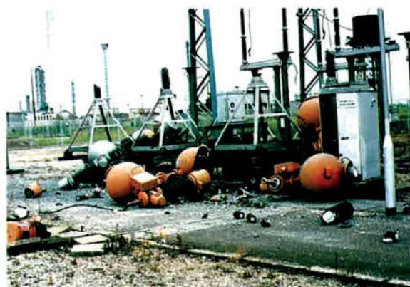
△ Switchyard of the Sisak thermal power plant after enemy attack
