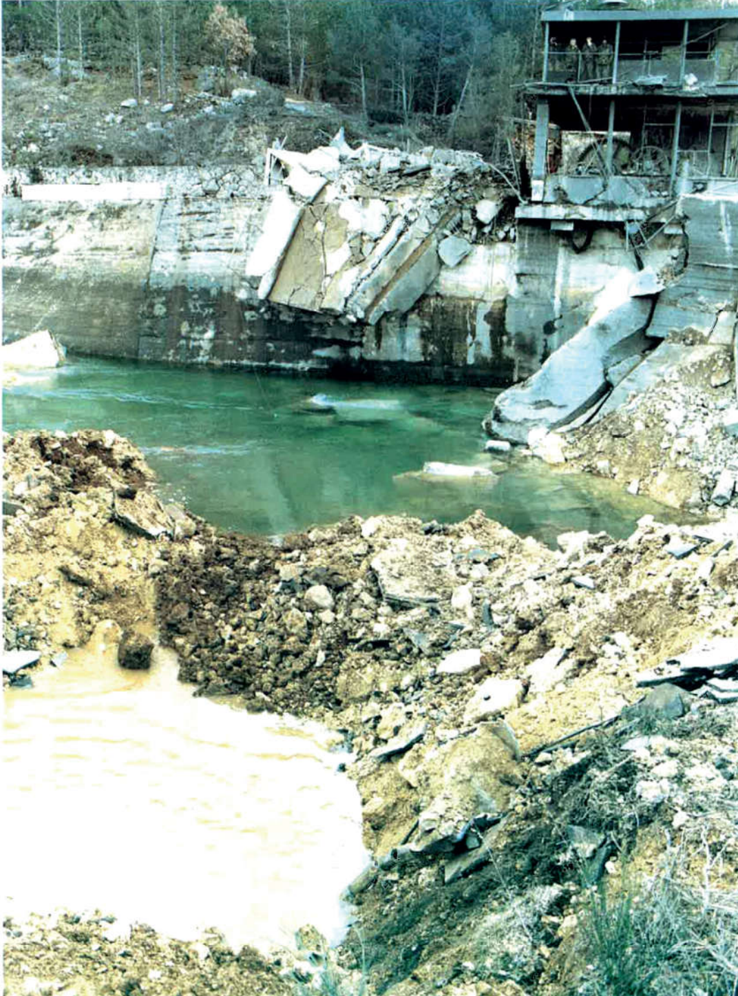
△ The Peruća dam, a day after being blasted, January 29, 1993
