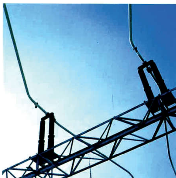
△ A detail of the 220 kV network
