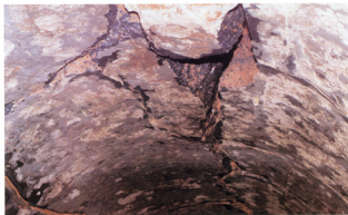
Cracks in the gallery arch concrete.
