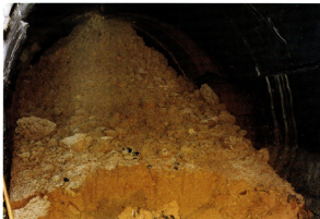
Photo 11. Caved-in gallery in station 3+42.00
