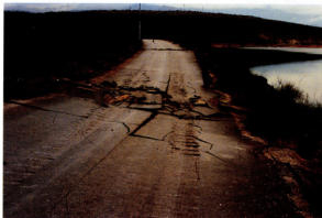
Photo 5. Crest subsidence in the highest dam section
