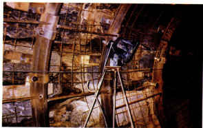
Photos 13 and 14 Concrete lining damage in the central grouting gallery section
