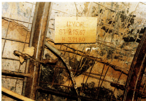
Photo 22. Water seepage into the gallery, El. 321.80
