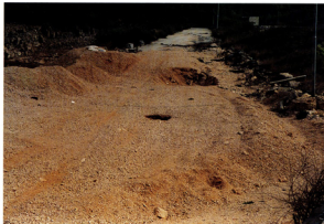
Photo 24. A view from the right dam flank towards the craters in station 3+62.00 formed on May 2, 1993 and 3+42.00 formed on June 3, 1993
