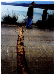
Photo 3. Transverse crack in the dam crest
