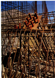
Photo 3. Flap bearing anchors and anchor plates
