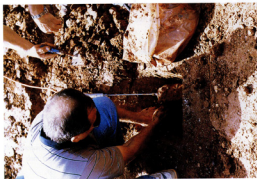
Photo 8. Total pressure cell placement
