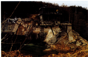
Photo 1. Spillway after explosion
