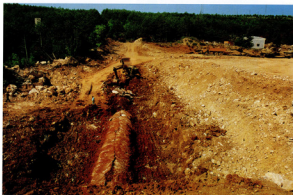
Photo 27. July 2, 1994 Right dam end - damaged grouting gallery top from the station 3+42.00
