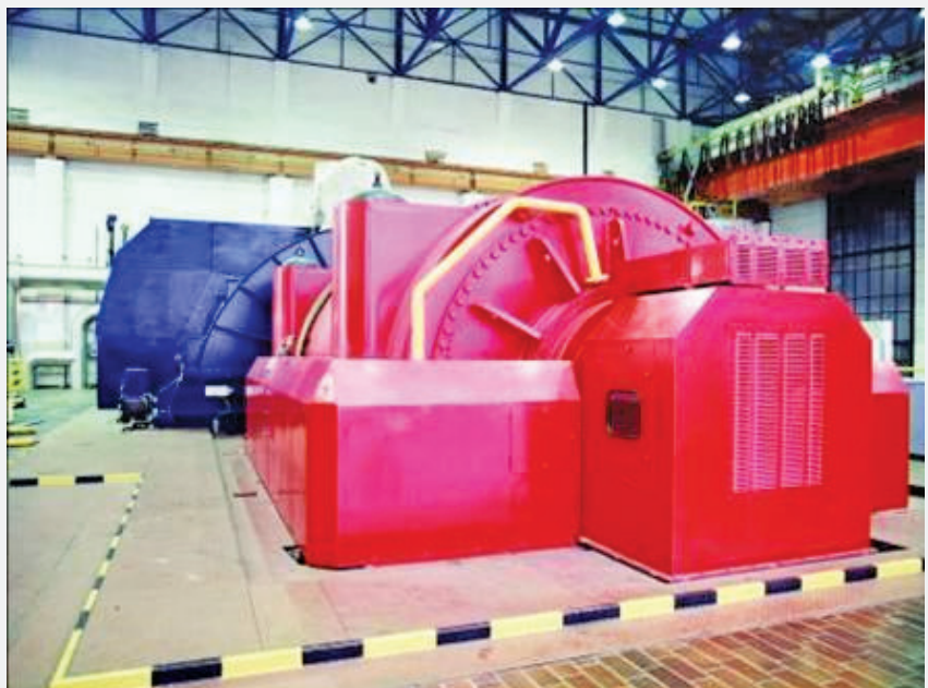
Turbogenerator snage 247 MVA instaliran u TE PLOMIN 2
