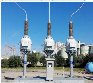
Inductive Transformer (step-up)
