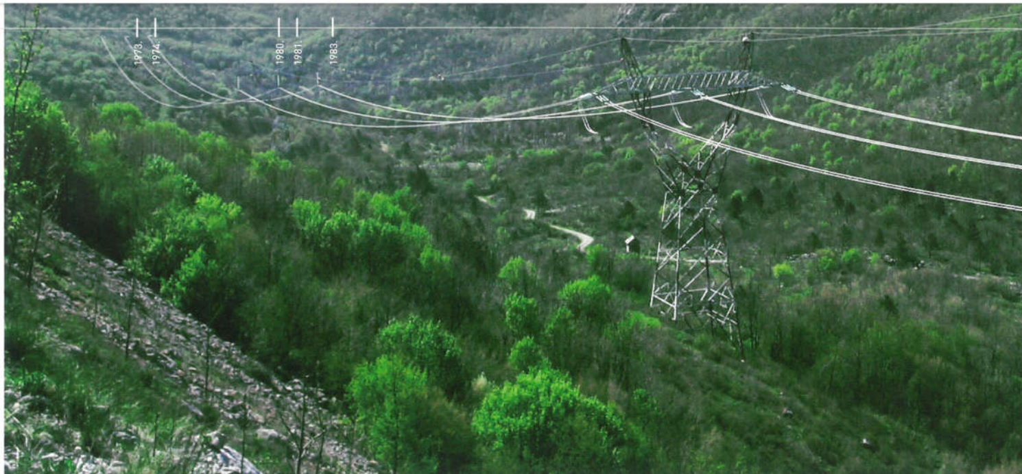
Trasa dalekovoda 400 kV Melina-Divača
