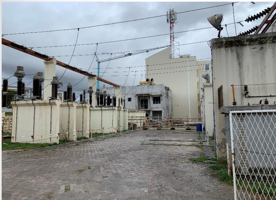
TS 110/20(10) kV Visoka
