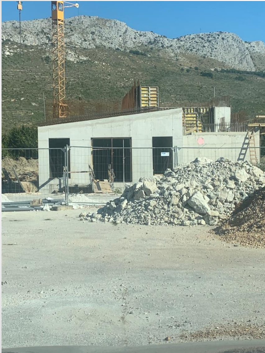
TS 110/20(10) kV Terminal
