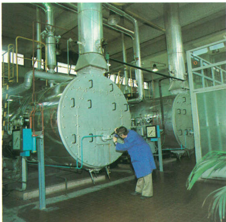
Plant for technological steam production
