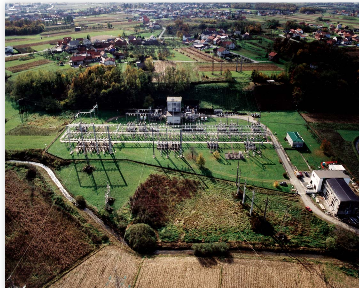
Transformatorska stanica 110/10(20)kV Rakitje
