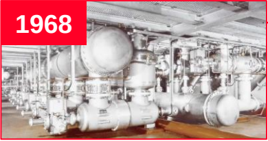
Gas-insulated switchgear (GIS) 170 kV
