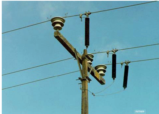
Figure 2 – Line arresters installed on 34.5 kV line – CEMIG [1]
