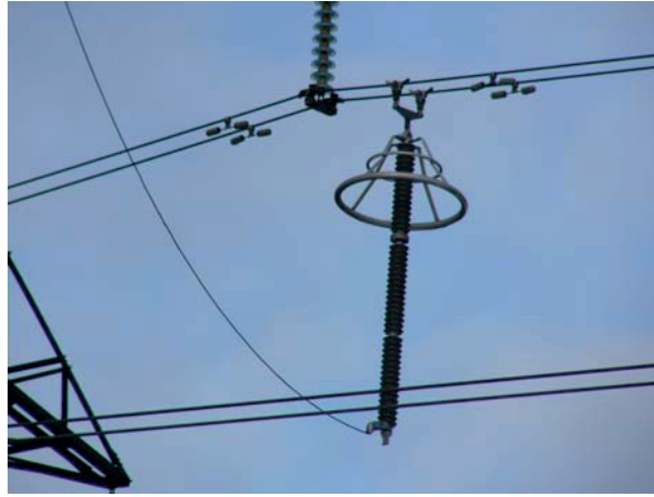
Figure 6. 400 kV line arrester in bottom phase.
