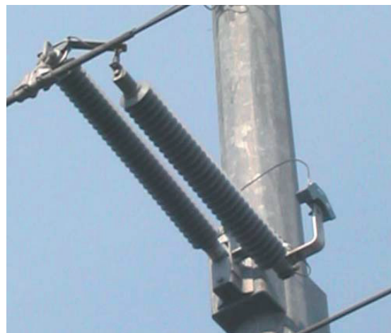
b) LSA installation (FPL)
