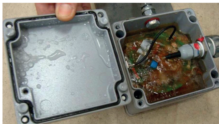
Figure 12 – Problem of water penetration
