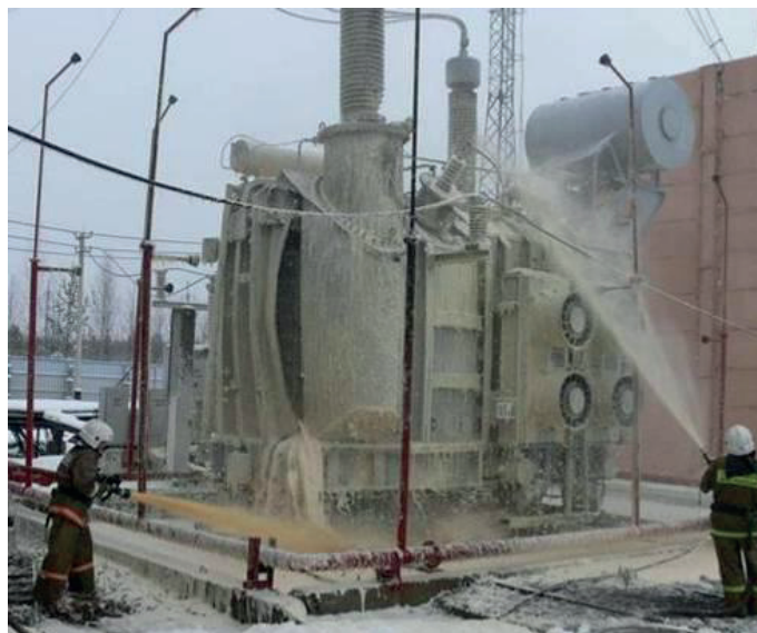
Figure 4 – Transformer in Western Siberia Substation after explosion
