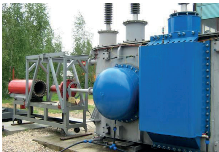
Figure 7 – Autotransformer with DPS before tests
