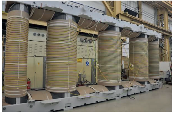
Figure 1 - Custom-made temporary windings during measurements
