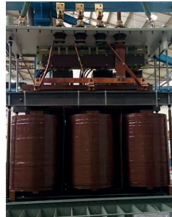
Figure 5 – RDT after short circuit test
