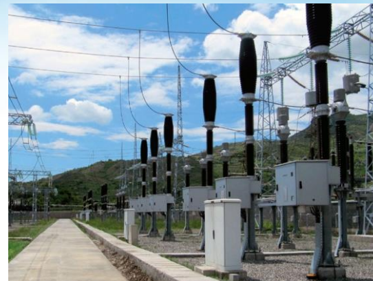
TS ELBASAN 1 220/110/35 kV Albanija
