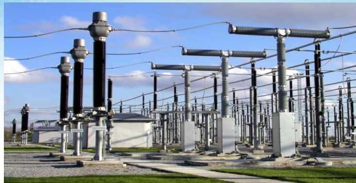
TS ERNESTINOVO 400/110/35 kV
