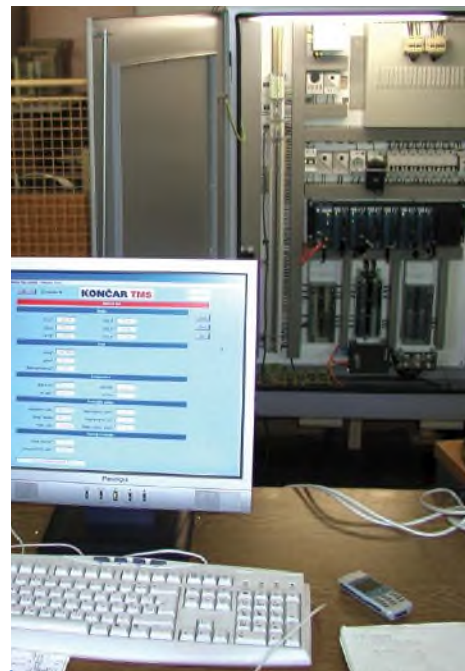
Monitoring sustav transformatora, 2006.
