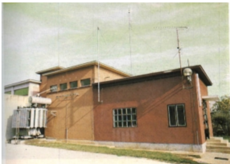
TS 35/10 kV Poreč I'
