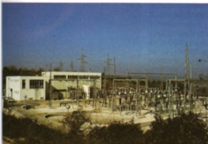
TS 110/35 kV Rovinj
