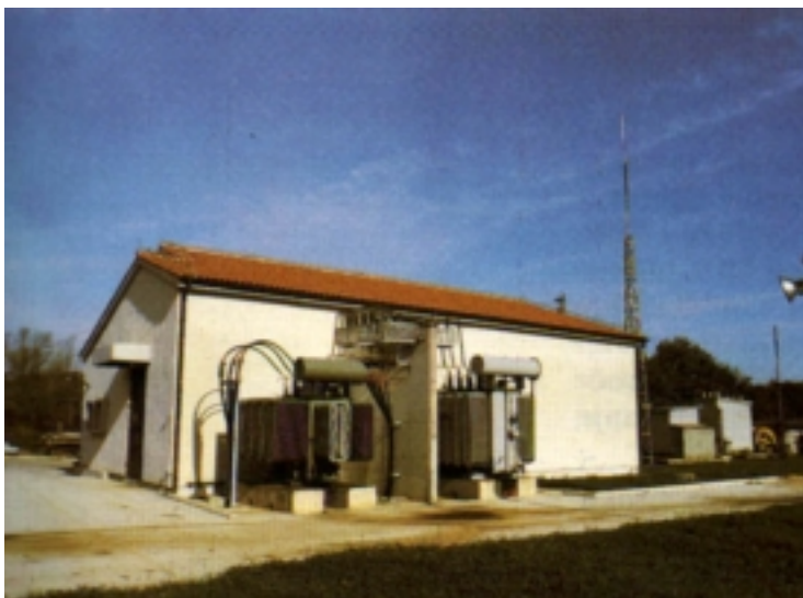
TS 35/10 kV Poreč 2.
