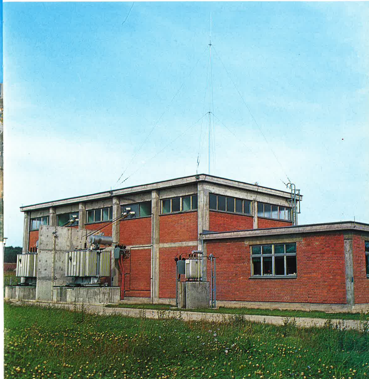
TS 35/10 kV Osijek — Retfala
