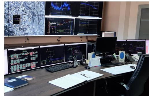
SCADA/DMS/OMS sustav u JP EP HZHB, BiH
