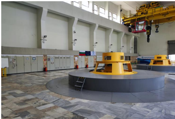
HE Momina Klisura, 2x60 MW
