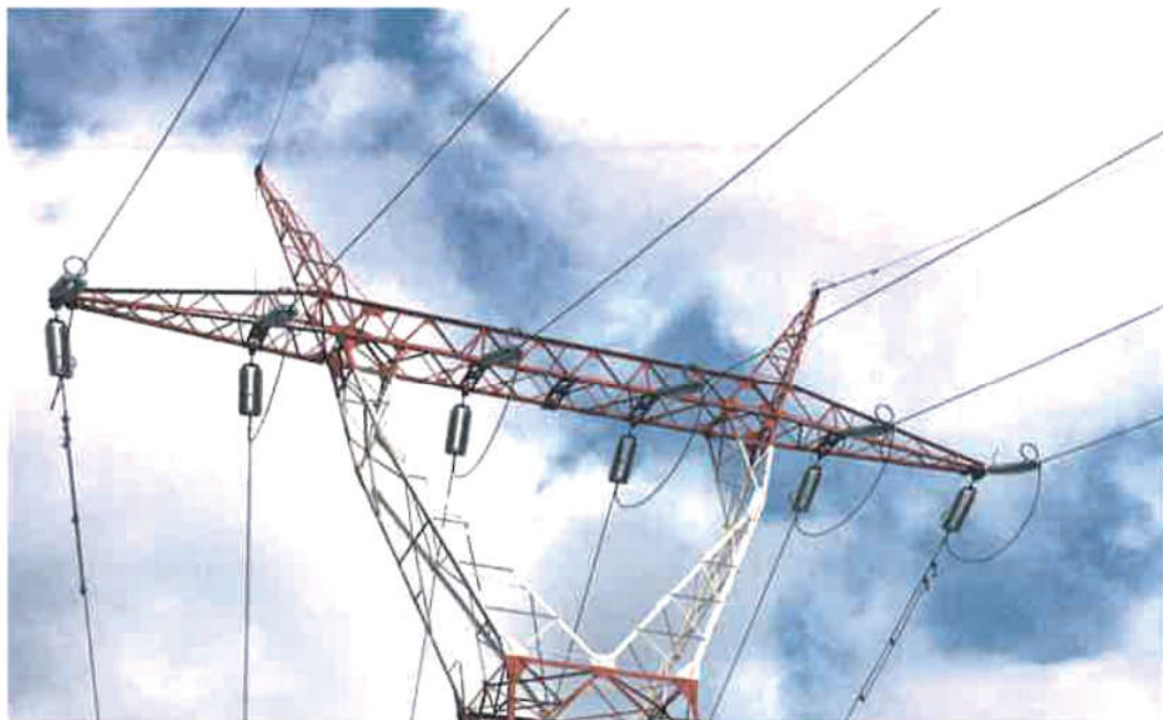
220 kV lines approaching Custóias substation
