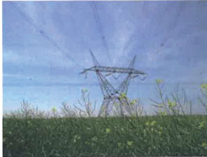
500-kV line, Alberta
