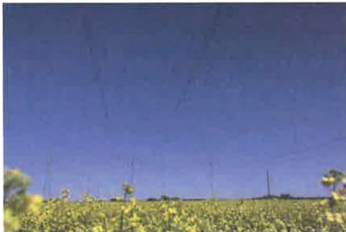
[Manitoba Hydro's HVDC Towers located near Gross Isle, Manitoba. Image courtesy of Manitoba Hydro / Mario Palumbo CPA.]
