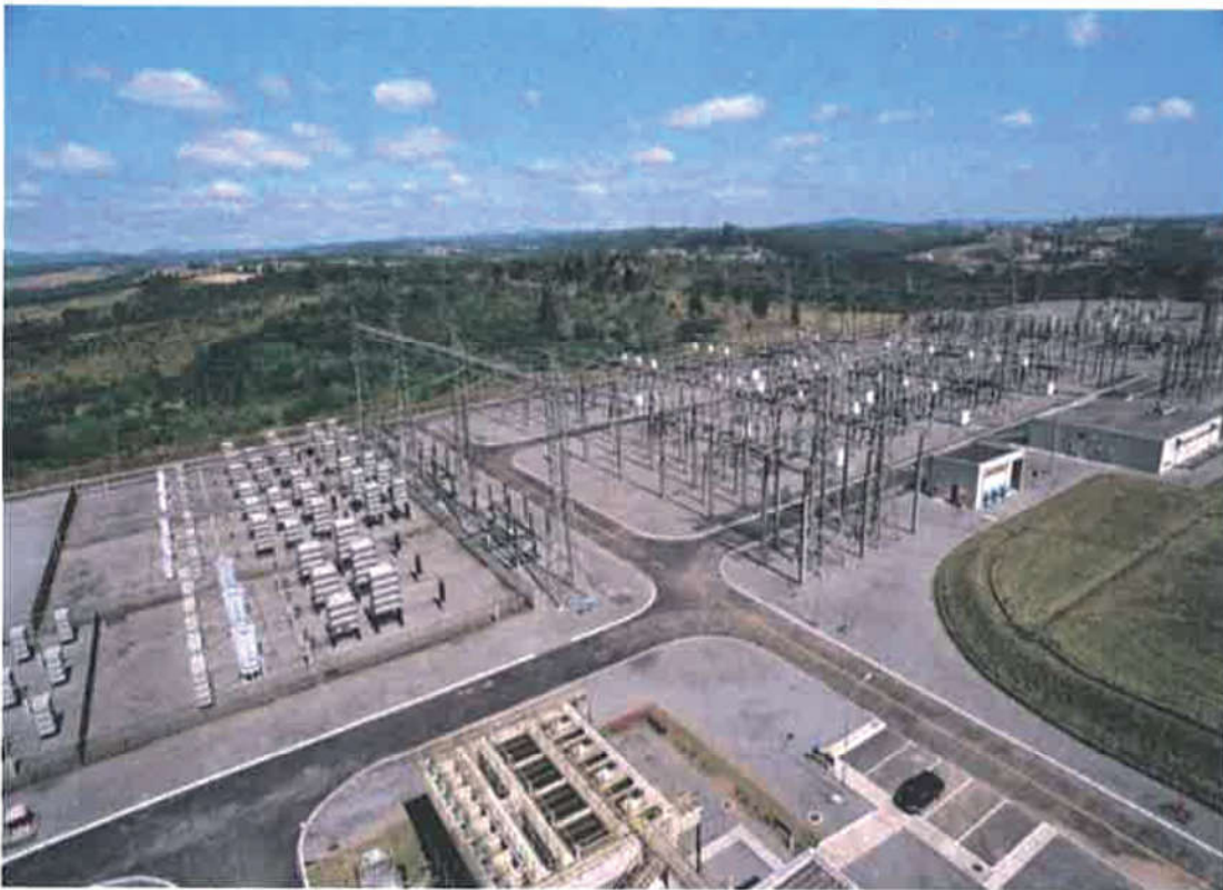
Ibiuna +/- 600 kV Converter station (Itaipu system)
