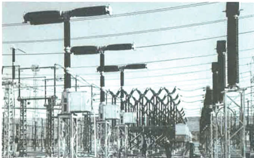
Fig. 3: 420 kV substation (1985) with minimum oil circuit breakers and SF 6 circuit breakers with two breaking chambers, both with spring-loaded drive. (Source: Areva)
