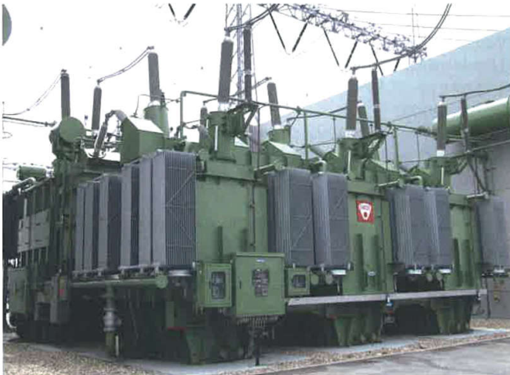
400/150 kV, 450 MVA shifting autotransformer at Pedralva substation
