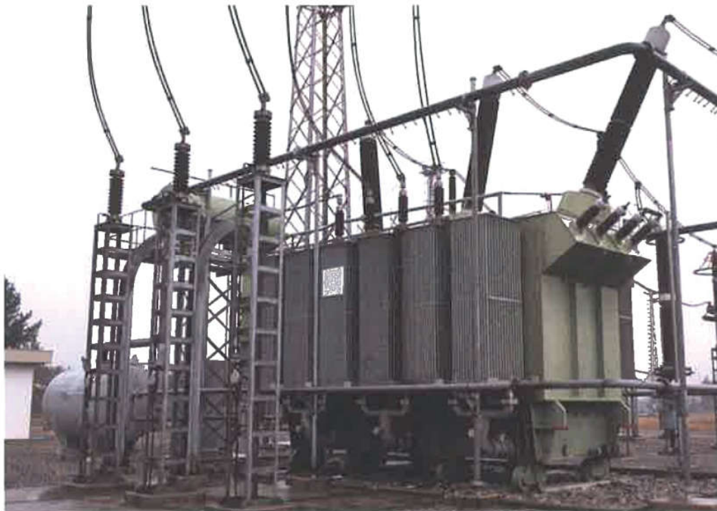
400/60 kV, 170 MVA transformer at Riba d'Ave
