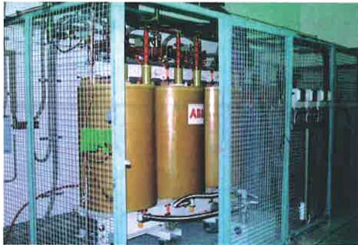
Fig. 6: HTS transformer station (630 kVA, 18000/420 V) at a SIG plant in Geneva. (Source: ABB Sécheron)
