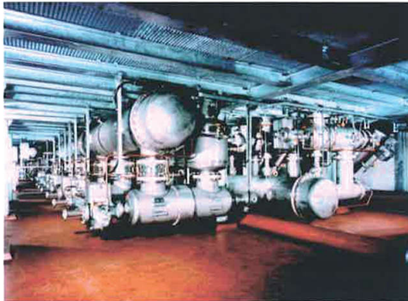
Fig. 4: Switzerland's first 125 kV GIS system at the Sempersteig substation in 1965. (Source: ABB)
