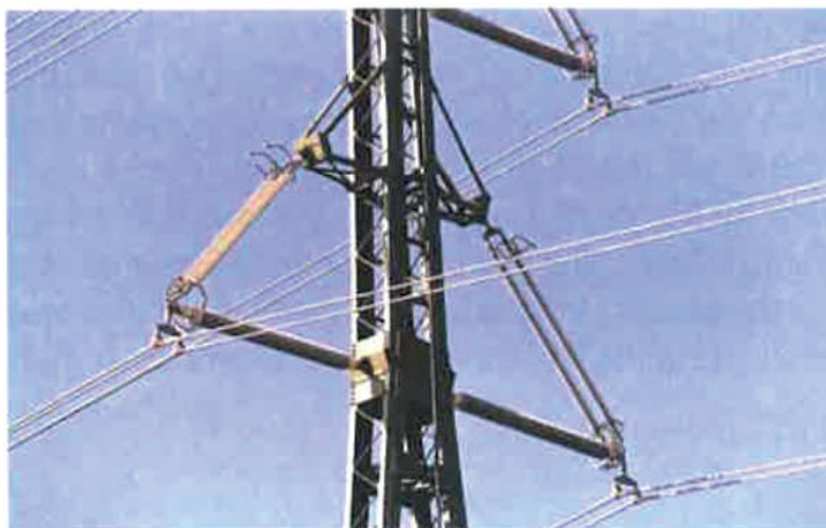
Fig. 7: Braced line posts on the compact 420 kV line near Lausanne. (Source: EOS)
