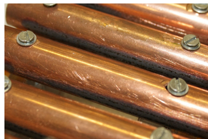
Figure 4.24: Heavy corrosion between the copper tubes.
